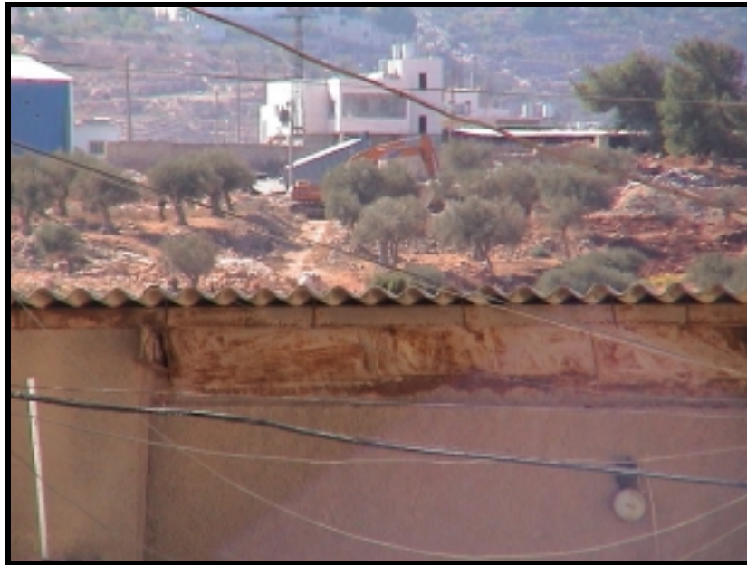
Photos 7 & 8 show the start of work of the segregation wall near Rachel’s Tomb 20/10/2003
