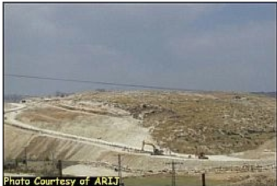
Photo 5 & Photo 6: Work continues in the Segregation Wall East of Beit Sahour, Bethlehem Governorate, ARIJ, and August 2003
