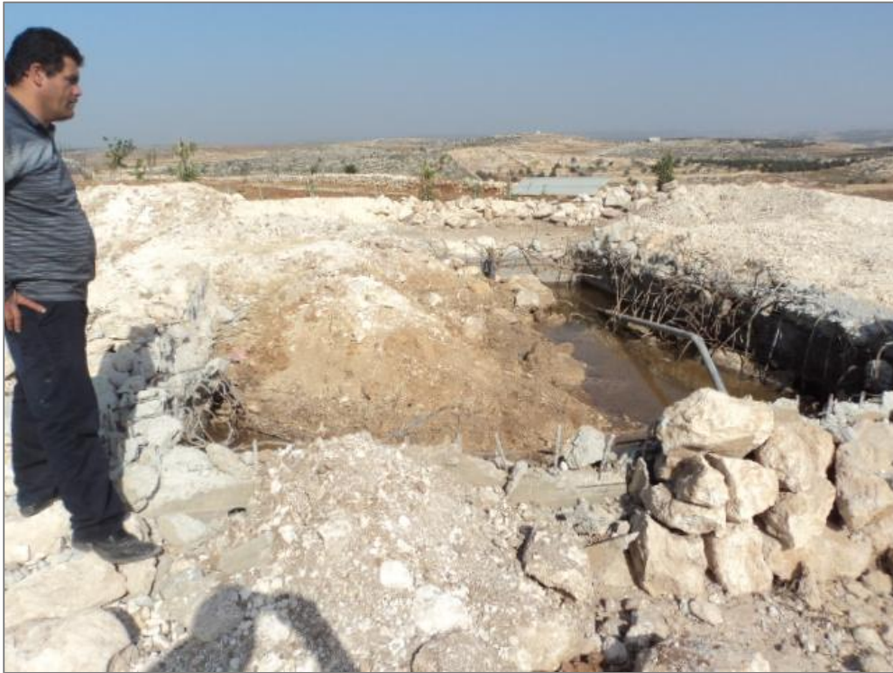
Photo 2: Demolished water well
