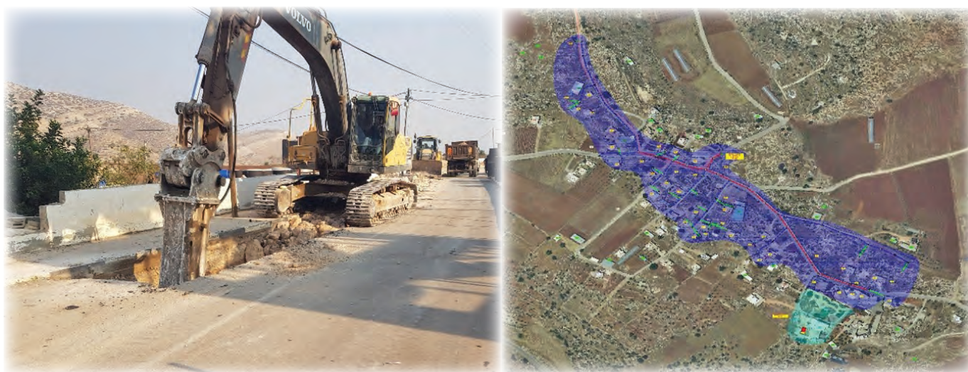
The sewage network and household connection at Al Aqaba- Tubas
